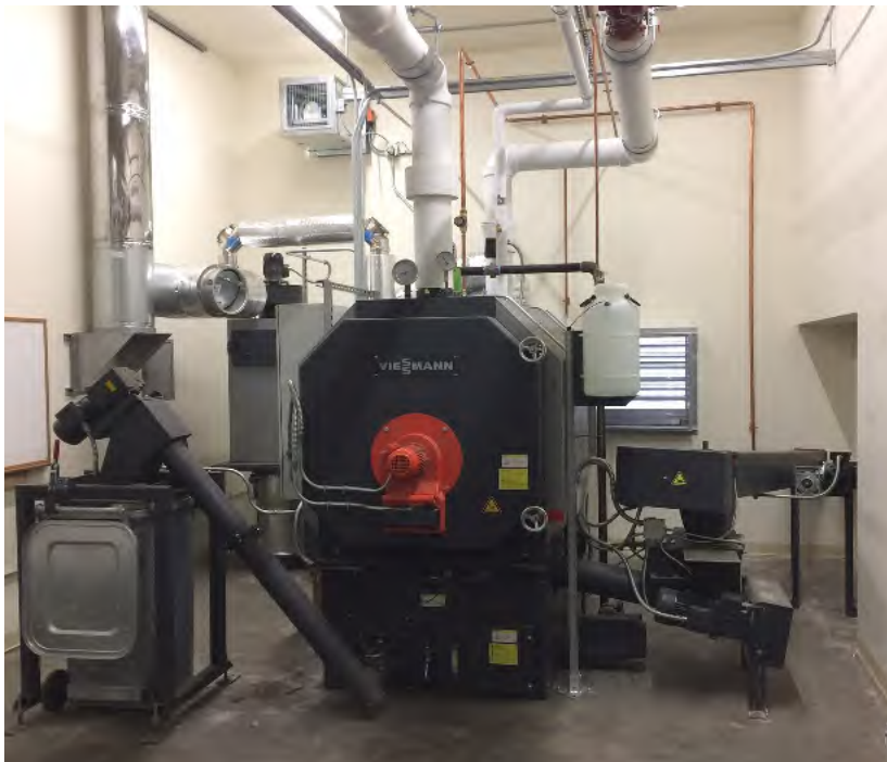
This biomass boiler features automatic ash extraction, a touch screen control panel, and a cyclone that keeps particulate emissions within NHDES limits.
