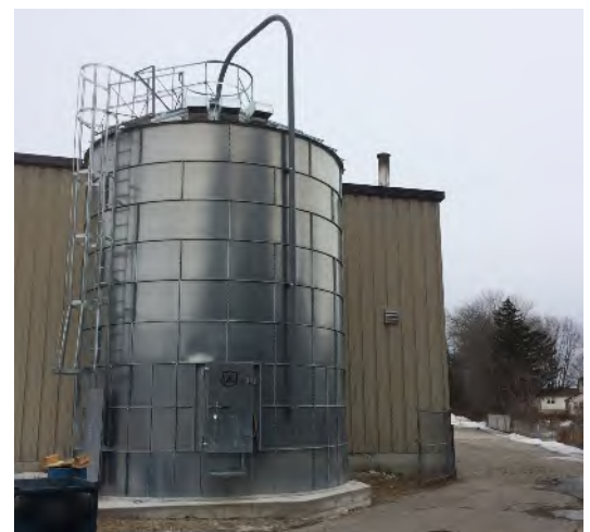
The 42 ton silo sits just a few feet from the new boiler room. PDCs are automatically augered directly into the boiler.
